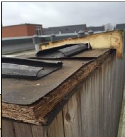
Linden fixed roofs to this cheap interior grade chipboard, one roof plunged 40ft writing off a car parked underneath.
