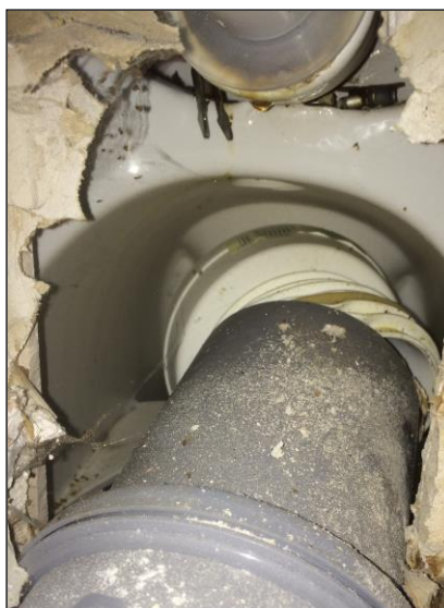
Linden failed to join this toilet waste pipe, so for months raw sewage was discharged straight into the building wall cavity.
